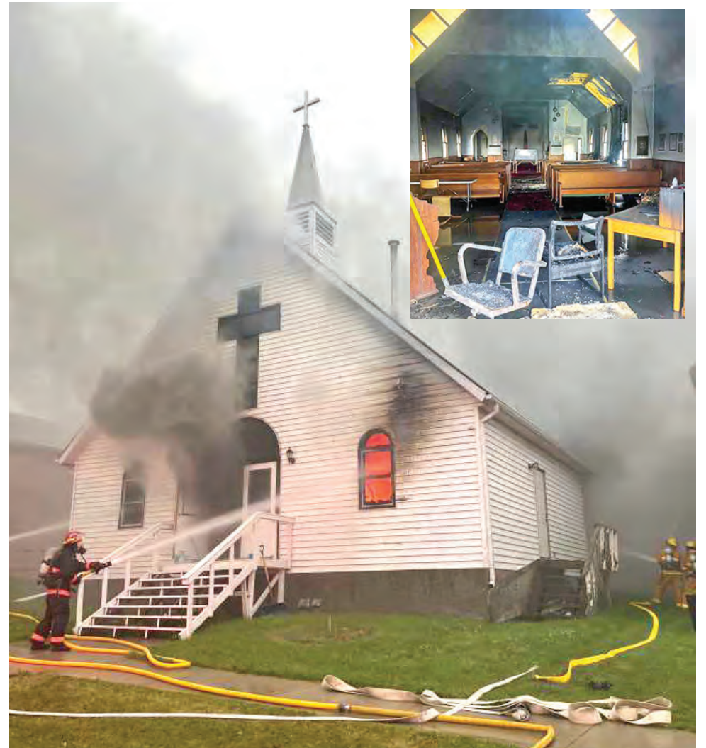
An early morning fire on July 1, 2023 caused substantial damage to St. Andrew's Anglican Church in Lac La Biche. Photos: RCMP
